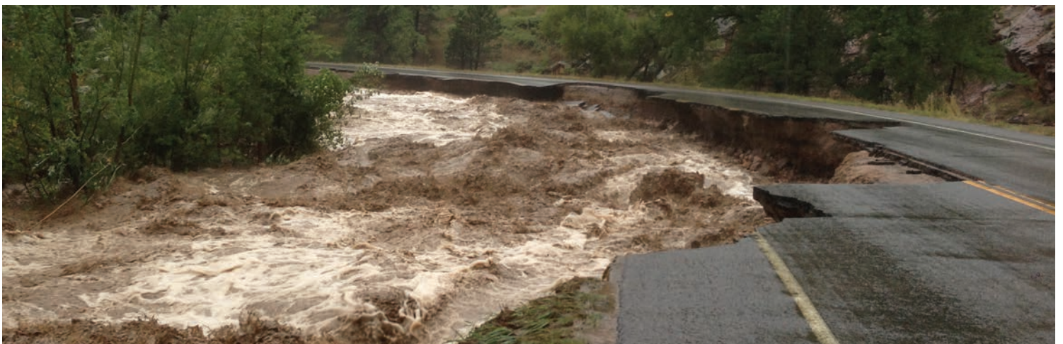
Lefthand Canyon Road with only a shoulder remaining for rescue access.
